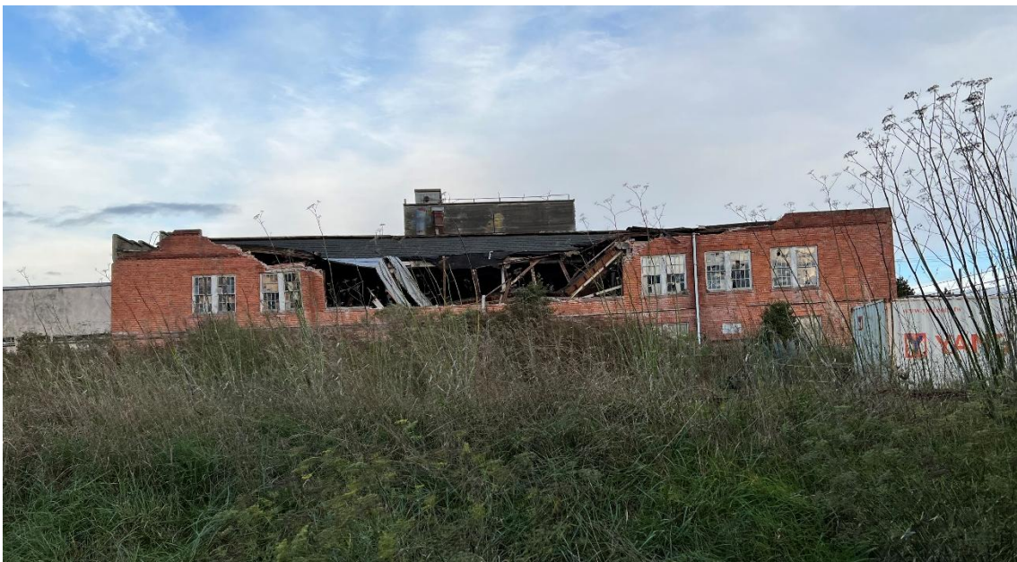
Figure 37: Earthquake Damage to a Brick Building in Humboldt County, 2021
