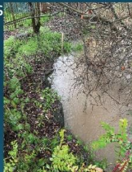
Upstream culvert outlet submerged and pressurized, tidal backwater
