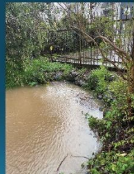
Downstream culvert outlet submerged, tidal backwater
