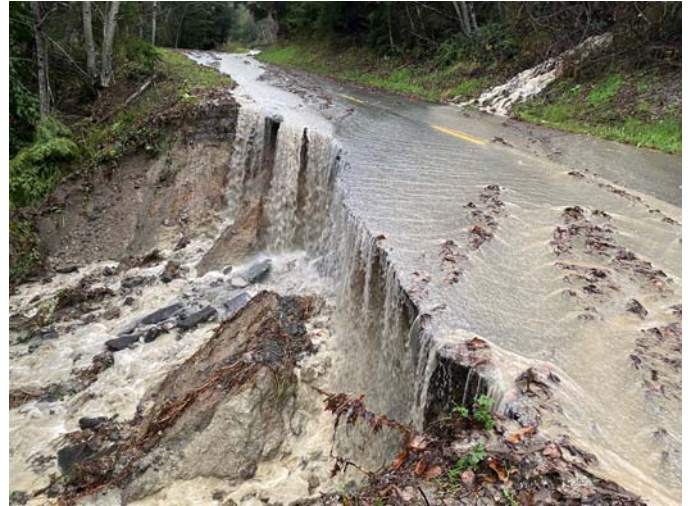
Flood damage sustained on Bair Rd. in January 2024.
