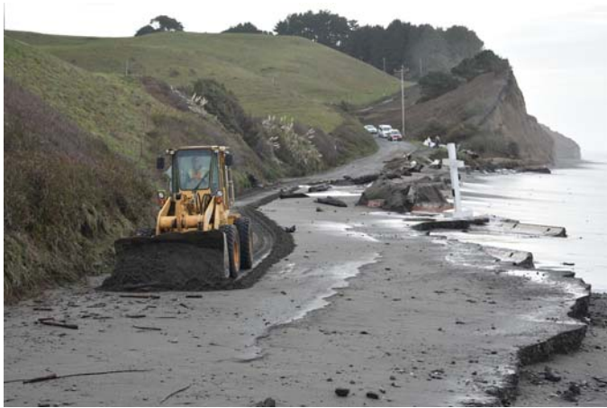
A Humboldt County Public Works roads crew works to repair Centerville Rd. in Dec. 2023.
