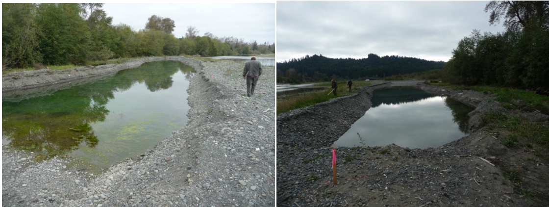
Figure 1. Alcove excavated in 2013 at the Guynup Site, Mad River. Left photo is looking downstream, right is looking upstream (photo date Oct. 11, 2013).
